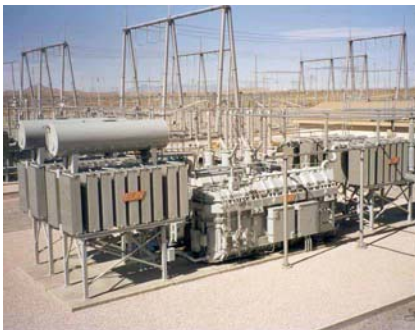
672 MVA/550kV Phase shifting transformer
